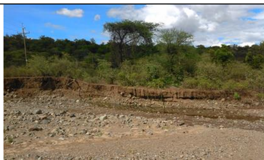
Plate 7.2 (c ): Erosion and deposits on a seasonal arm of the Perkerra
