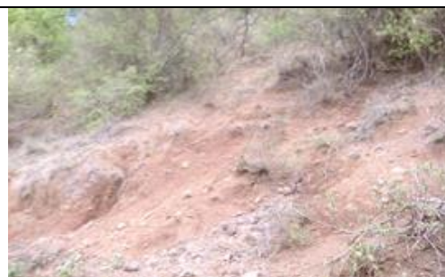
Plate 7.2 (d): Erosion on degraded hill slopes in the project area
